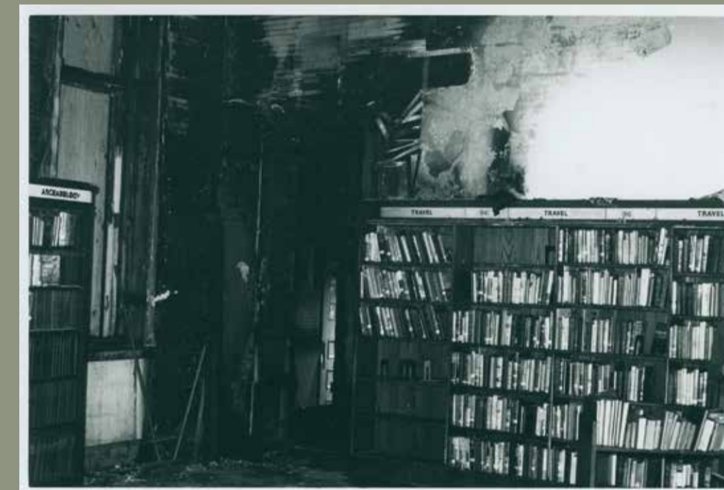
Damage after fire on 10 November 1969 Vandals lit fires in the children's storyroom and in the workroom, causing $35,000 in damages and the destruction of 2,000 books.
